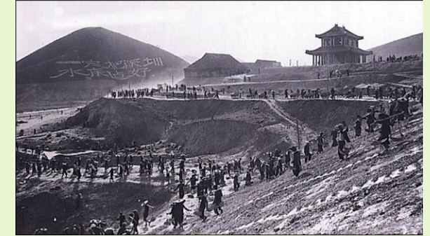
Shenzhen Reservoir was an important source of water supply for Hong Kong. The photo shows the construction of Shenzhen Reservoir in 1959.
